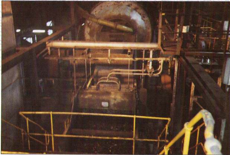
Far Left: Surface Loading Point. Left: Coal Preparation Plant.
